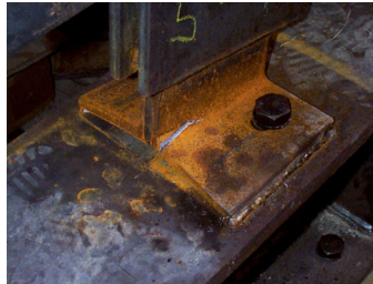
Cracking of angles
