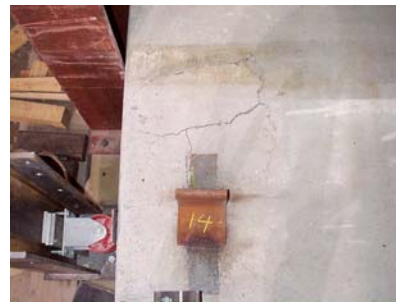
Typical failure away from plank end
