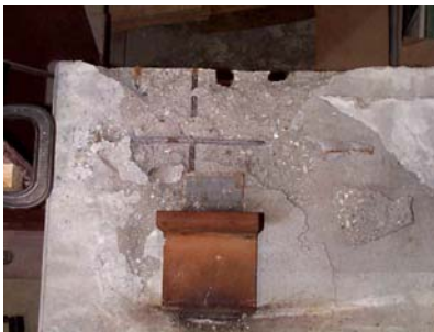
Typical failure at plank end
